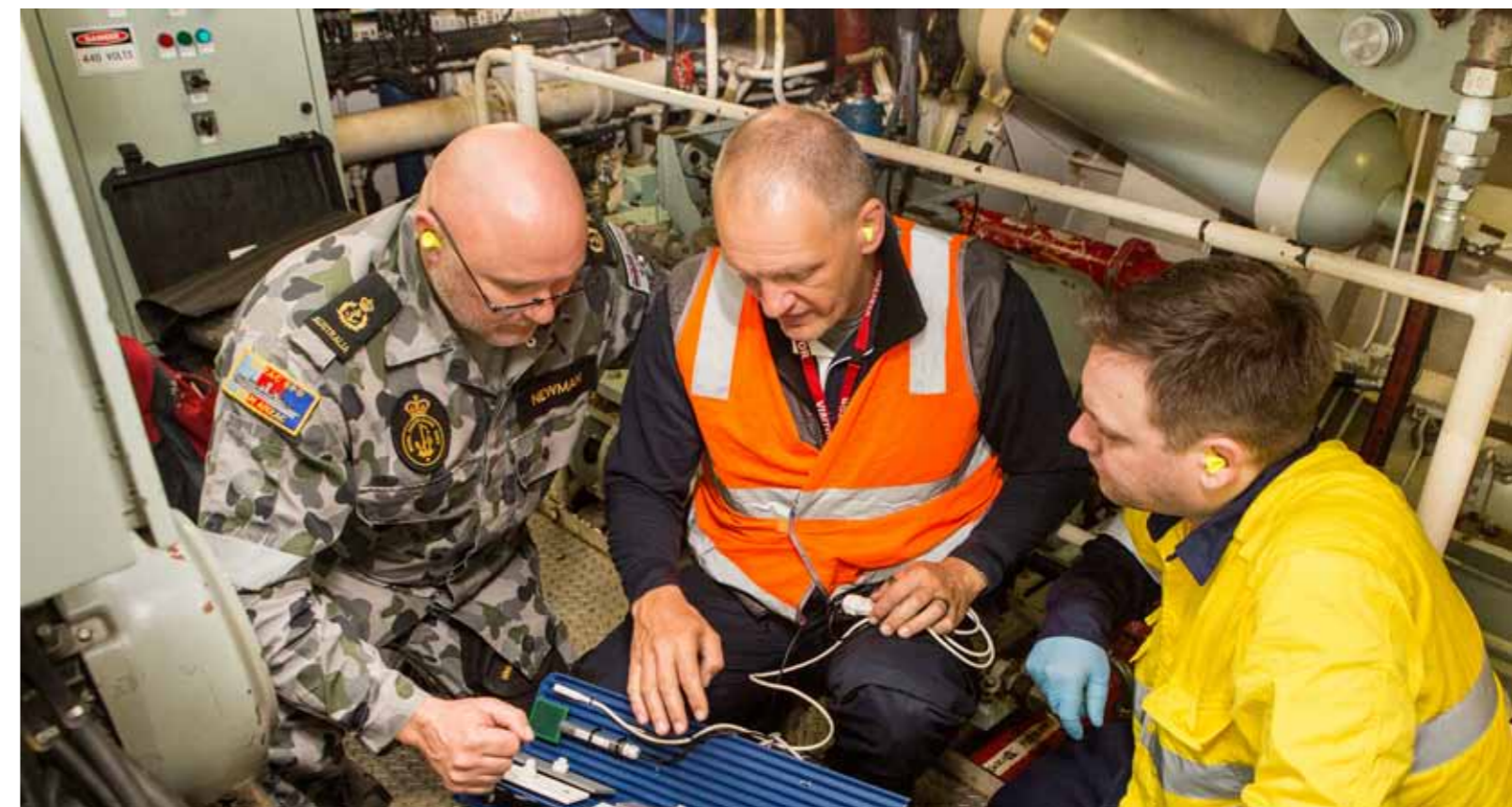
Assoc Prof Geoffrey Will, QUT, (centre) and Dr Steven Knight, SUT (right) show Marine Technician CPO Todd Newman (left), how the corrosion prognostic monitoring system works during the systems installation in the Gas Turbine Machinery Room onboard HMAS Parramatta , Sydney.
